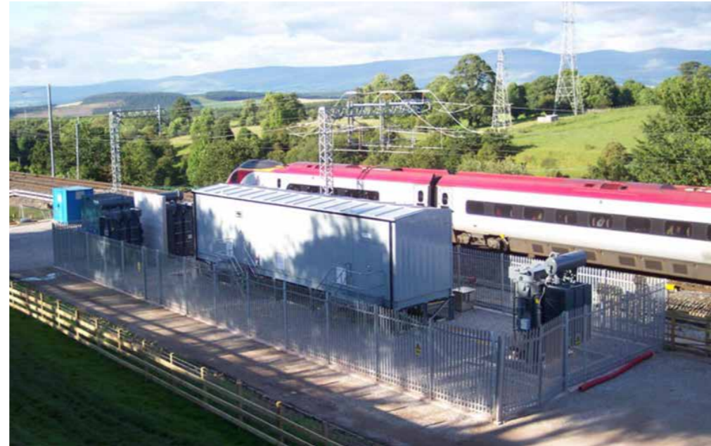
Intrusive Auto-transformer Station with harsh materials and fencing ©WJPServices
