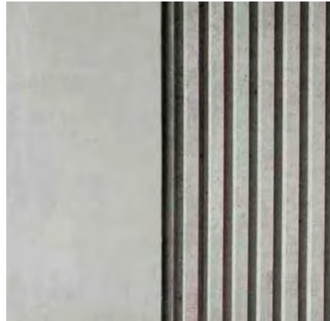
Texture and shadow gaps mask joints and reduce mass of structures ©CRT
