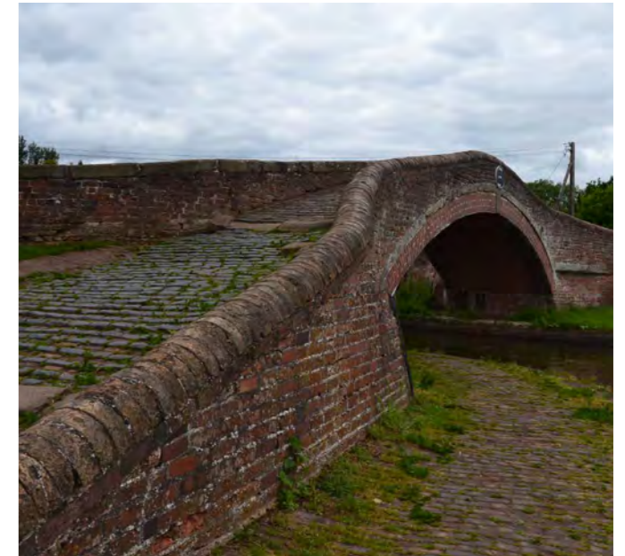
Haywood Bridge Scheduled Monument, with surviving historic materials to the bridge and surfaces
